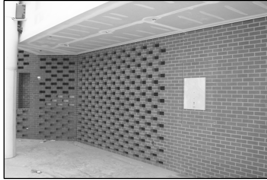
This is a back wall in the new worship space. The missing bricks are filled with material to assist in the acoustics. Also shown on the wall is a limestone mounting for our Stations of the Cross.
